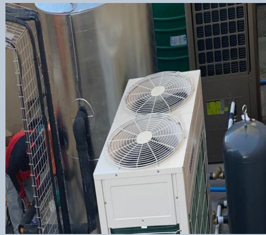
VRF/DVM Heat Recovery, Hot water heat pump plant - Mantsopa Specialised TB Hospital
