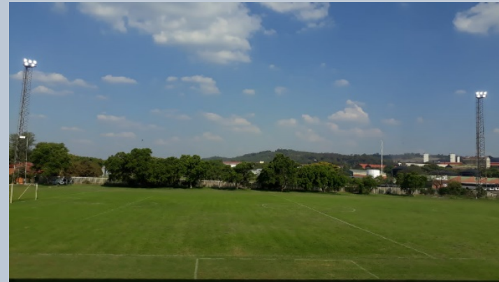
New LED Floodlights at Tshwane South TVET College Pretoria West Campus Stadium.
