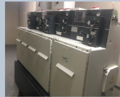
Substation switchgear service – Pareto PTY LTD, trading as Cresta Shopping Centre
