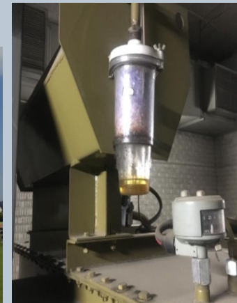
Transformer service - City of Johannesburg Metropolitan Head Office
